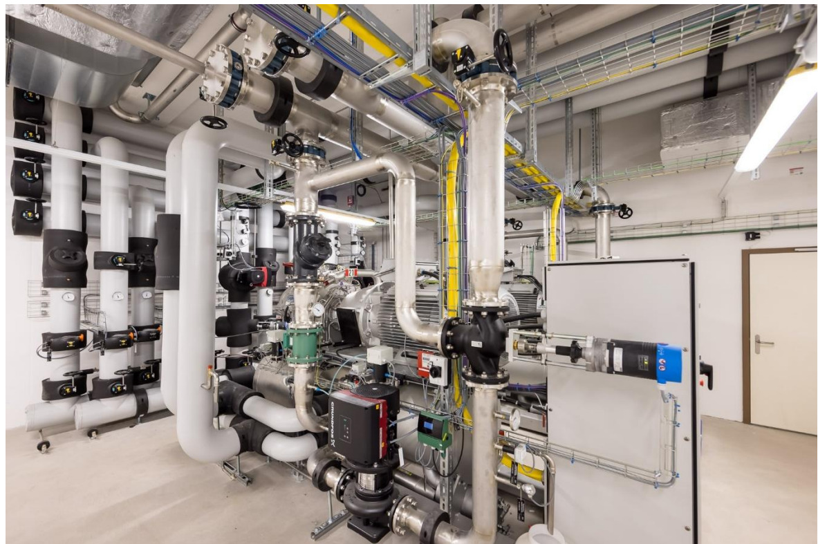
Chiller in the refrigeration center in the new building (2021)
