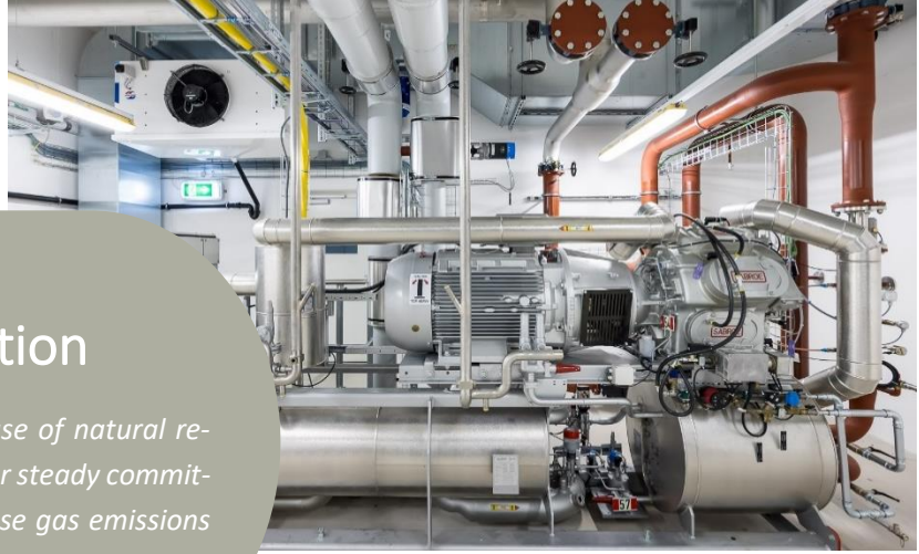
The heat pump in the energy center of Chocolat Bernrain, commissioned in 2021
