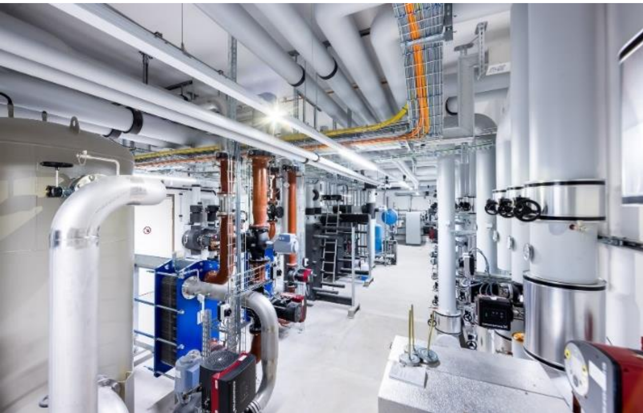
Heat and cold distribution in the Chocolat Bernrain underground
